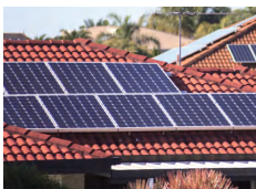
Solar panel Solar panel mounting
