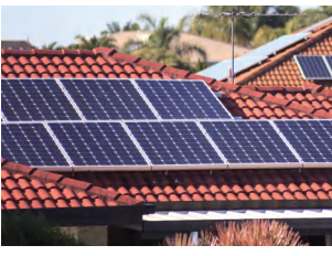
Solar panel Solar panel mounting
